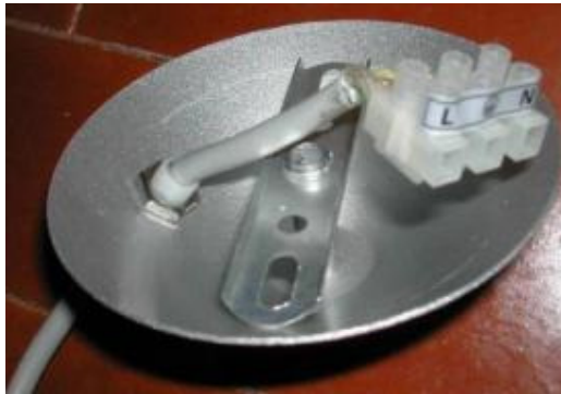
Example of metal part not connected to earth
