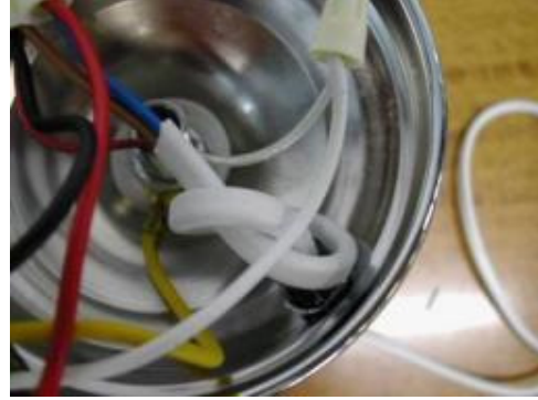
Missing cord anchorage for supply cable (knot is not allowed)
